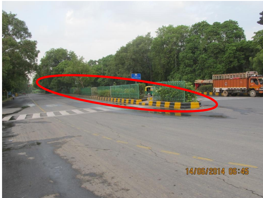
Figure 2.5: : Overgrown Suburbs at the Median Portion on the Aurobindo Marg Approach obscuring the visibility of the traffic emanating from Prithiviraj Road Approach until it reaches the mouth of the intersection (b)
